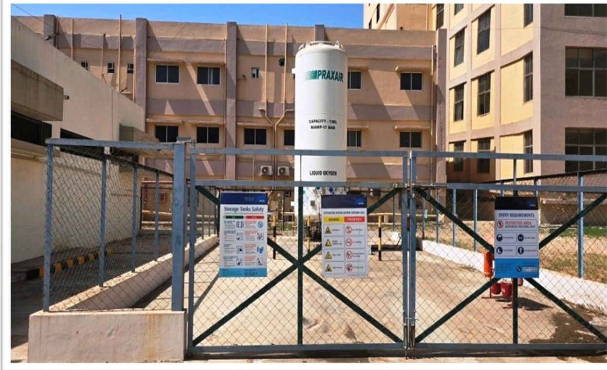
Liquid Oxygen Plant
